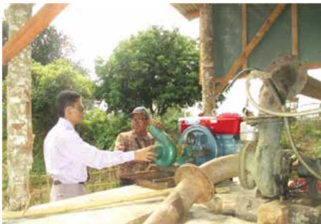
Figure 46: Power pump at Abinash para, Panchari
