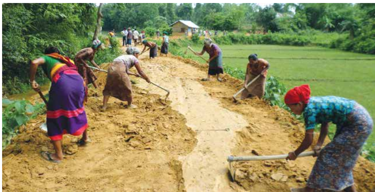
Figure 10 LCS women working to construct VAR at Dharmapur in Khagrachari sadar upazila
