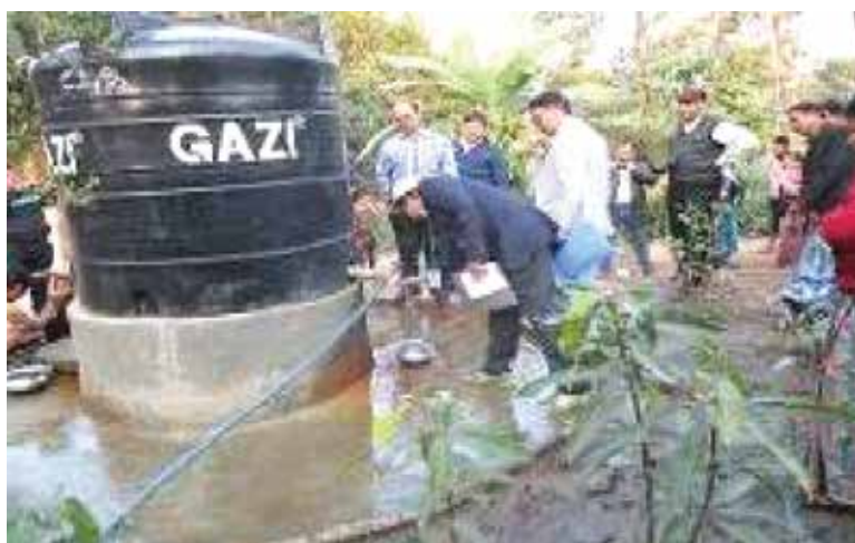
Figure 31 A water supply system at School para in Khagrachari Sadar Upazila
