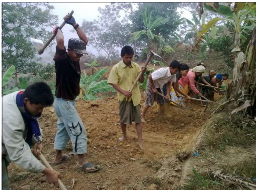
Villagers work together to build a new village path; we support communities to collectively bring changes to their lives
